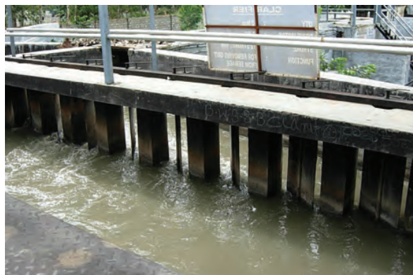
Fig. 13.4 Grit and sand removal tank
