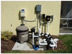
Fig. Water purification
