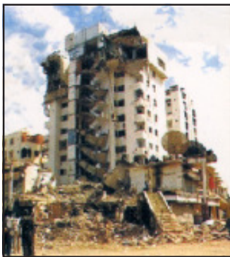
Fig. 3.3a: Destruction caused by an Earthquake in Gujarat
